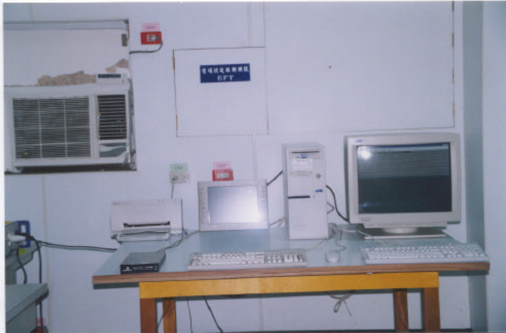
Power Line Test
