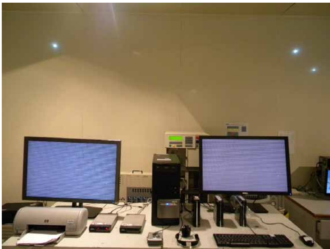
For Telecommunication port
