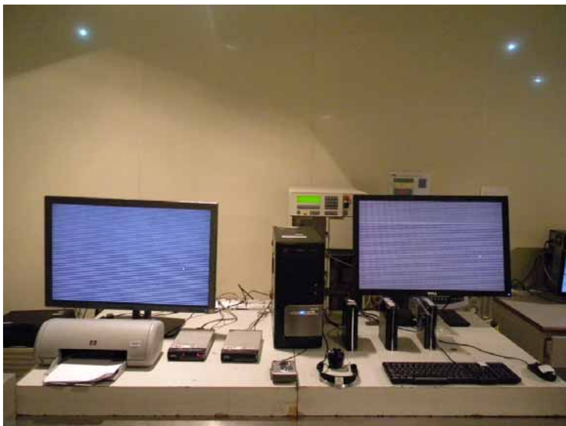
For Telecommunication port
